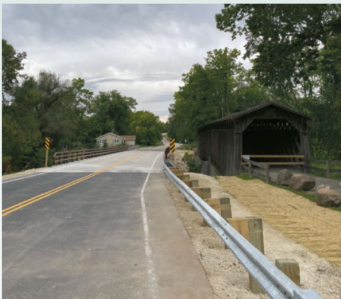
Photo Above: Covered Bridge following completion of total reconstruction in summer of 2022.
